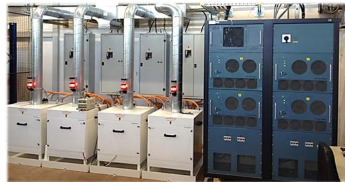
An ABB battery module testing facility
