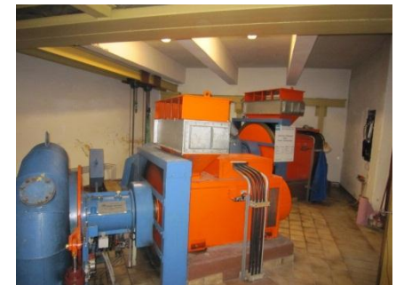
hydro power plant Graggaber (1,1 MW_EPL)
