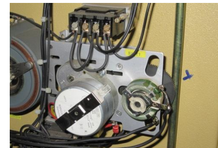
motor potentiometer hydro power plant Graggaber
