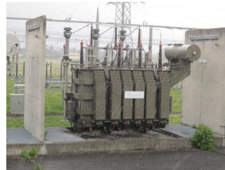
110/30-kV-transformer Lungau, 32 MVA
