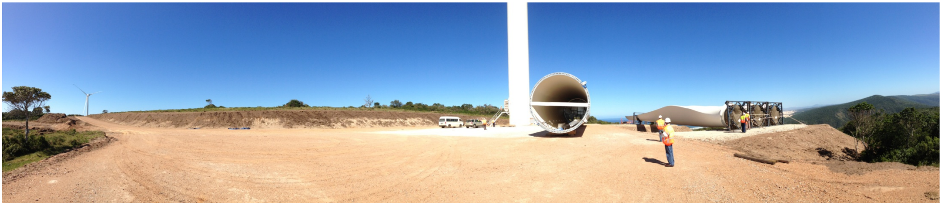
Van Staden's Wind farm, 27 MW – Round 1 project under REIPP
