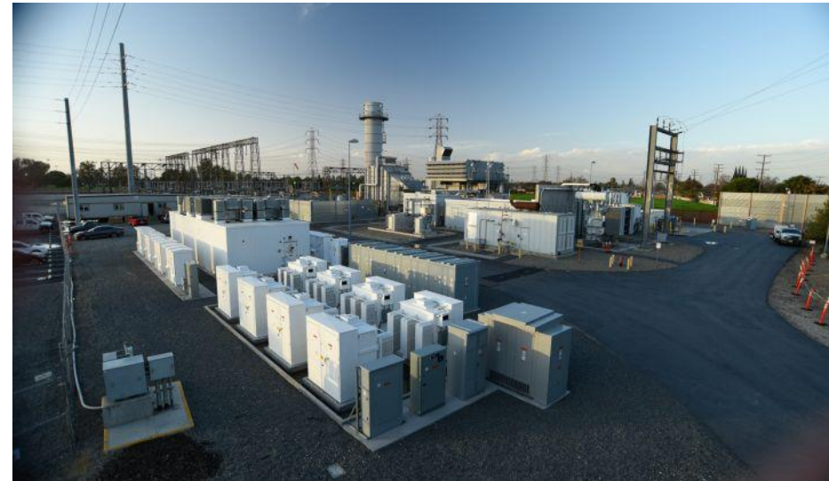
Southern California Edison hybrid battery storage, gas turbine peaker system
