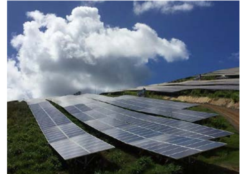
4.2 MW PV Array USVI Pre And Post Hurricane
