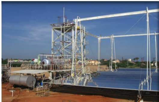
Solar steam generator with thermal energy storage for desalination
