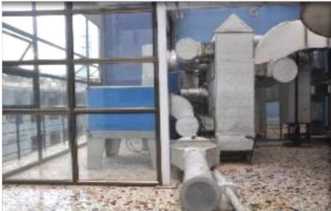
Dedicated outdoor air system (DOAS) technology testing at IIT Bombay
