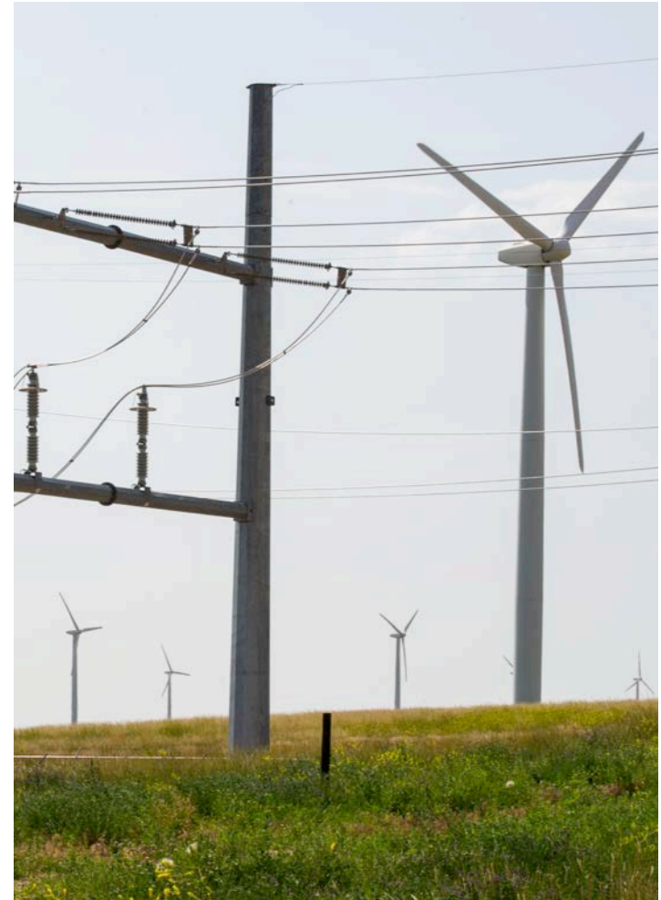
Source: Schroeder 2014 (NREL PIX 31732)
