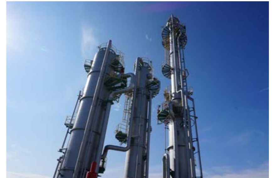
CO 2 Capture facilities
