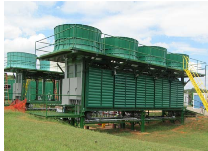
First Commercial Demo Plant GT DAC 4000
