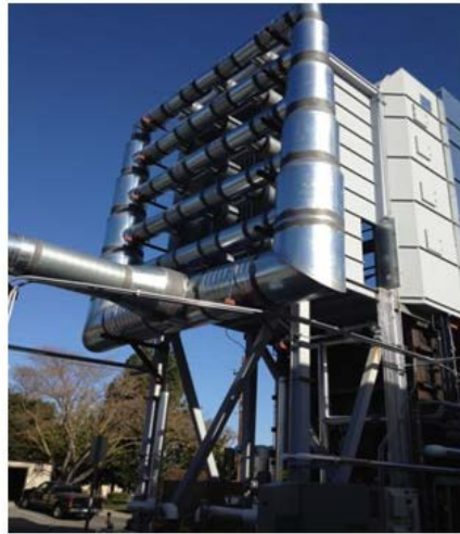
Second Pilot Plant GT DAC 2 / GT Carb 1
