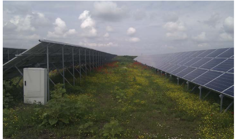
9.6 MW PV power plant
