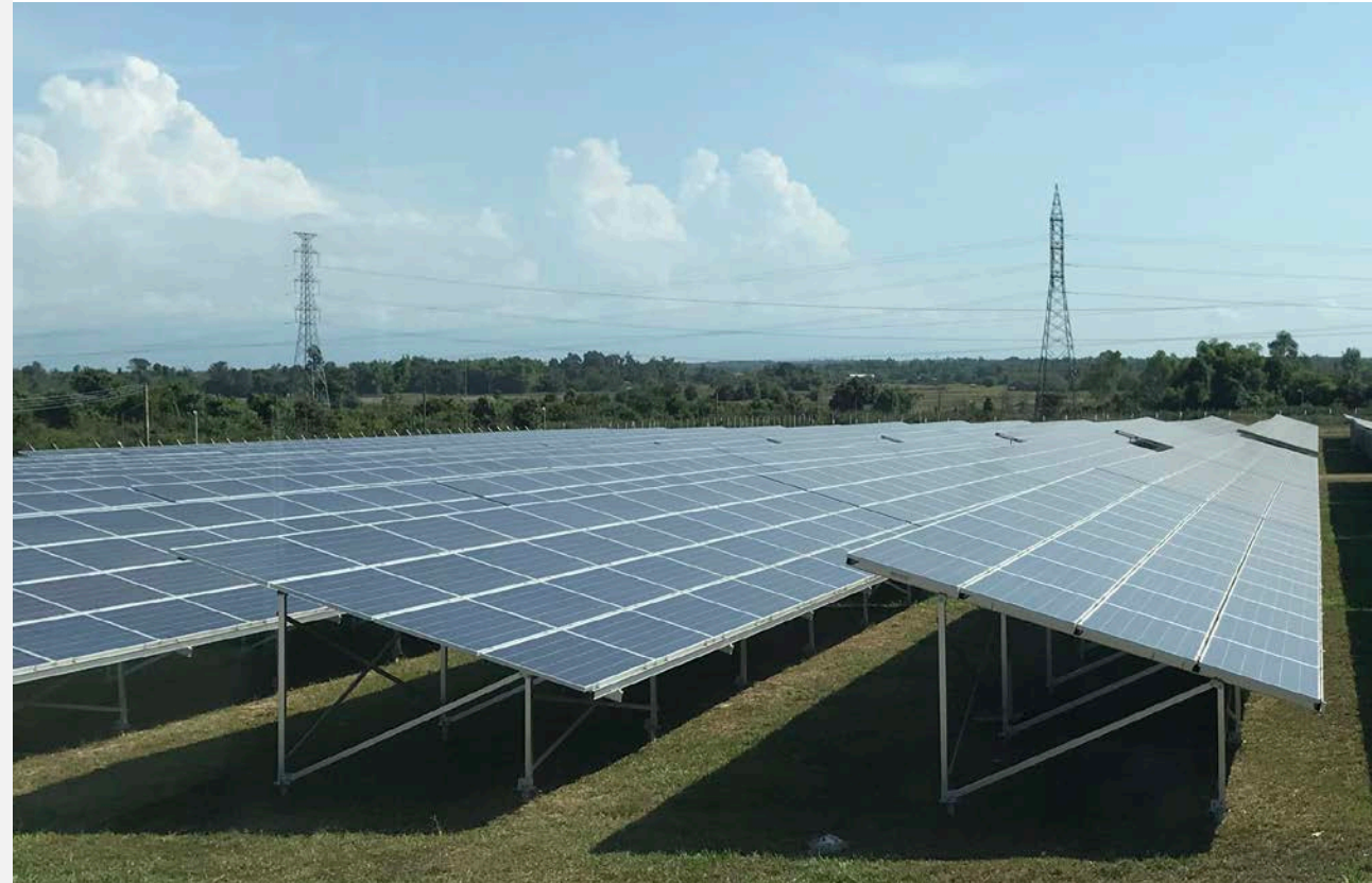
Figure. EDL-Gen Solar Photovoltaics Plant, Naxaithong district, Vientiane
